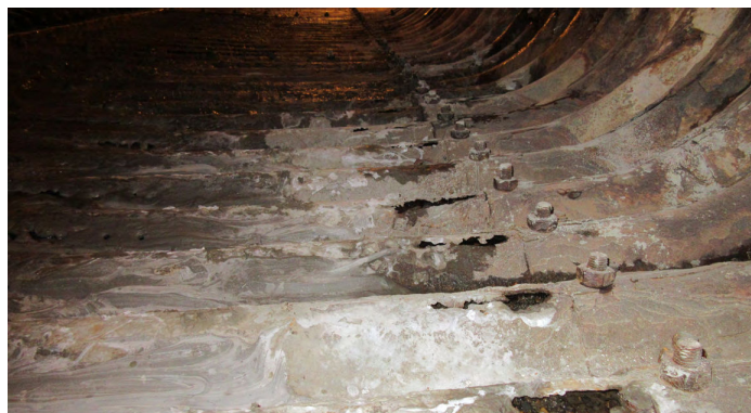
Filling of corrugations covering damage
