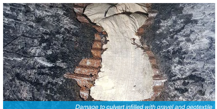
Damage to culvert infilled with gravel and geotextile
