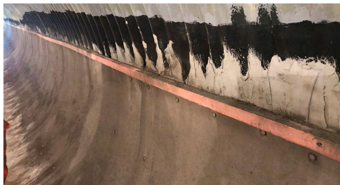
Timber secured to provide a cutting edge guide for a neat finish
